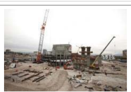
COURTESY SMITH CENTER FOR THE PERFORMING ARTS Whiting-Turner Contracting Co. recently topped out the $470 million, 170-foot-tall Smith Center for the Performing Arts, on 4.75 acres, at 361 Symphony Park Ave. In downtown Las Vegas. The project will take an estimated 1.5 million man-hours to complete by 2012.
